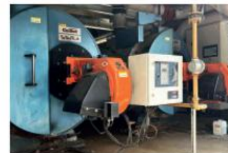
Boiler room n°3
