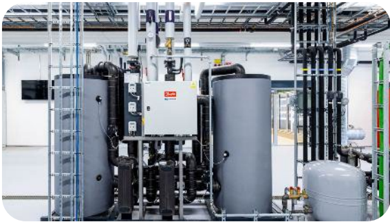
Heat Recovery Units
