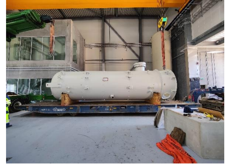
CO 2 storage tank
